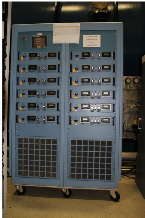
316 Automated Heater Controller
