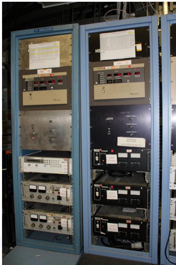
Electrical Heater Controller
