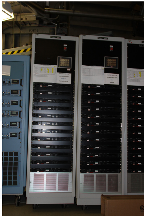
315 Automated Heater Controller
